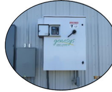
Variable speed drives on fans, separator and composter
